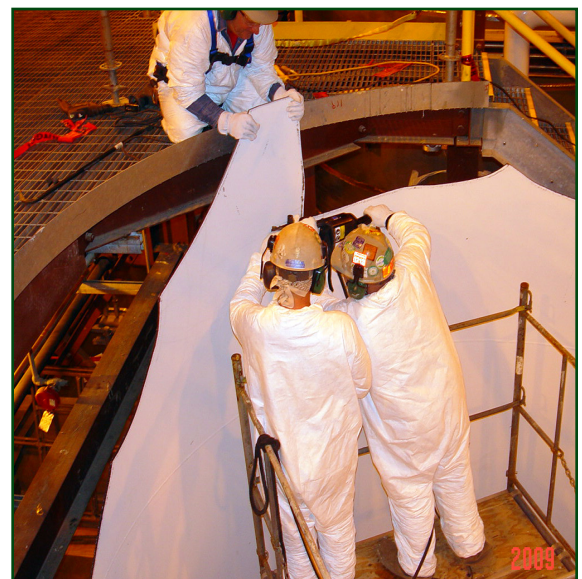
Workers removed the process auxiliary building (PAB) tank as part of phase one operations. The PAB will be demolished.
