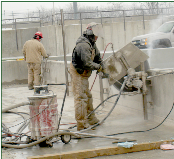
Employees are working at the Intermodal Storage Area located in the Chemical Limited Area at NECDF. Currently, this area is used for temporary storage of roll-off containers until off-site shipment for disposal.
